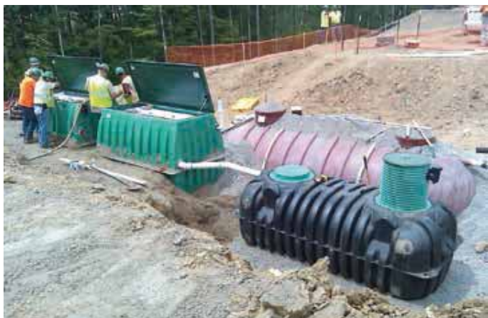
At the BSA's National Jamboree site, AdvanTex® Treatment Systems from Orenco treat up to 757,000 liters per day of graywater for reuse. Photo by Biohabitats, Inc.
